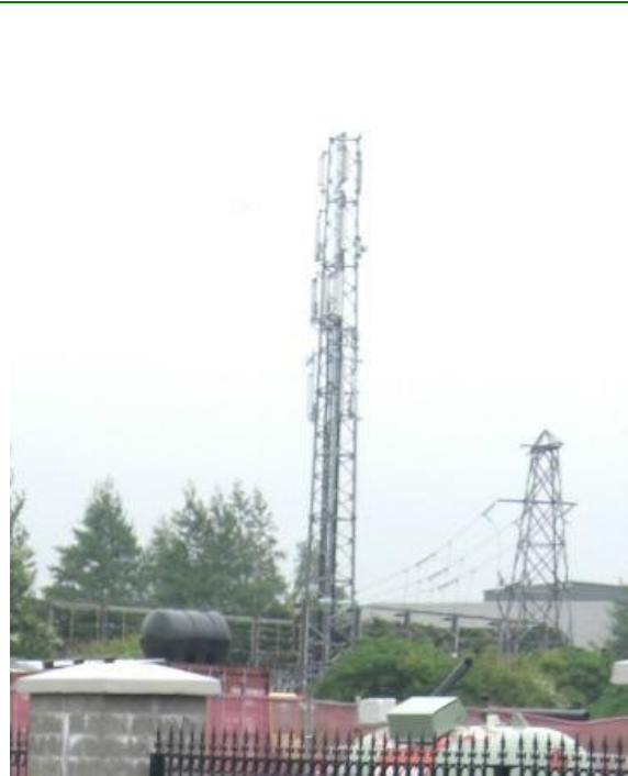
Transmitter Site Photo
